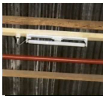
One of the six new electric lights
